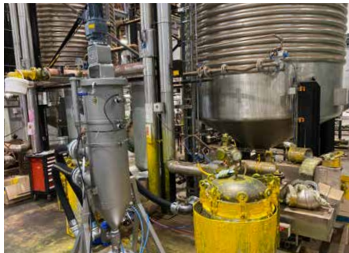
Auto-line XXL-E self-cleaning filter installed in the production and filtering ink.
