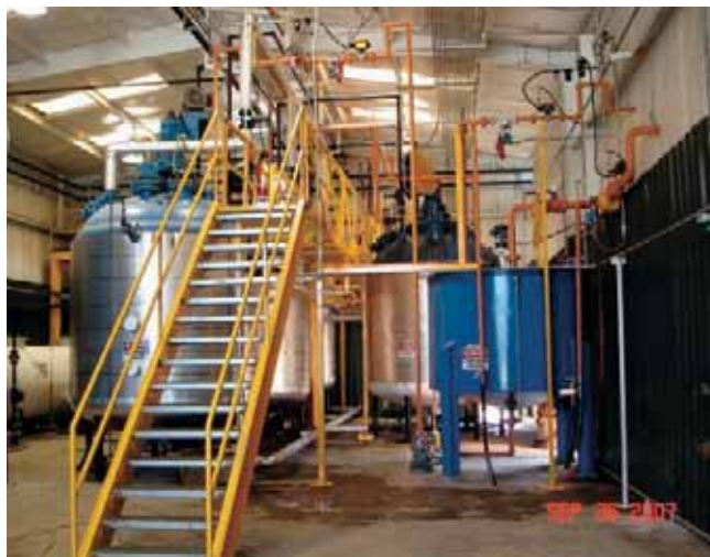
Figure 2. Interior view of Alterra Energy Facility
