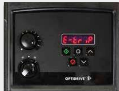
Local display of activated protection
