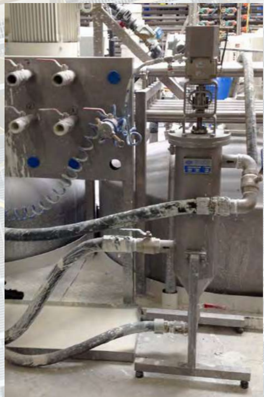
Larger filter installation for water based coatings
